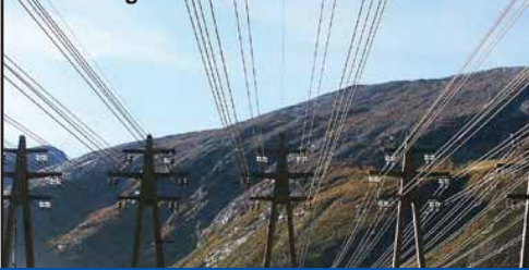
Power Line Monitoring
